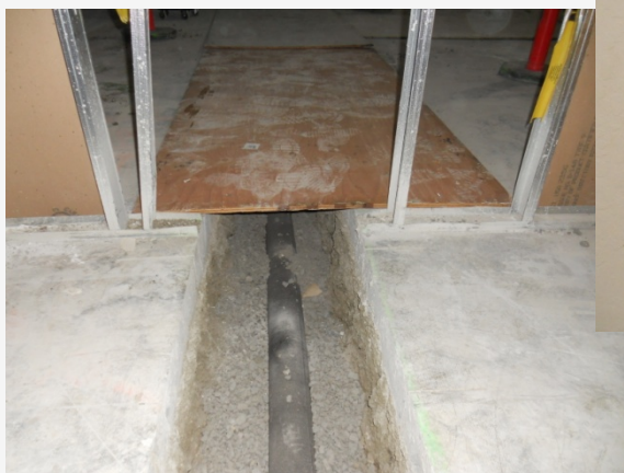
Sub-Slab Vent Pipe
