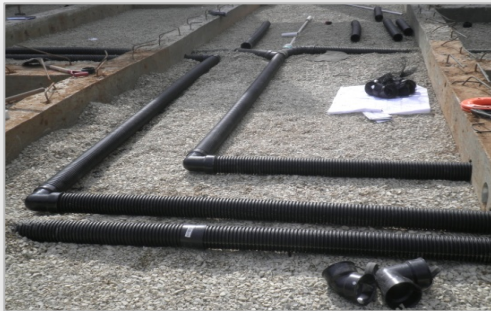
Sub-slab vent piping
