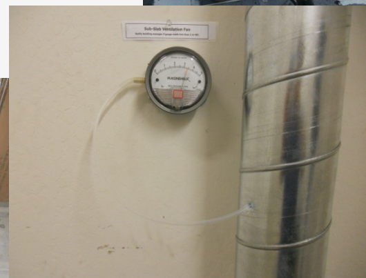
Riser Pipe; Vacuum Gauge
