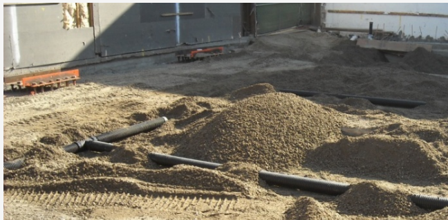
Sub-slab vent piping
