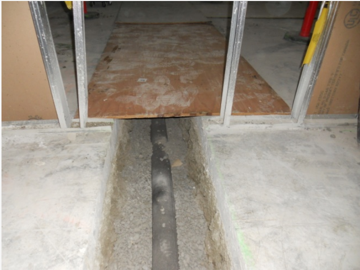
Sub-Slab Vent Pipe
