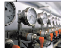
Pressure gauges at a wastewater treatment plant Photo: Dana Point Times/Andrea Papagaris
