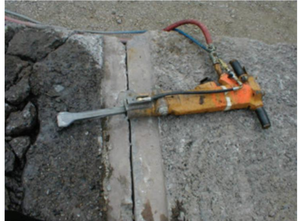
Jackhammer equipped with water spray delivery system to control dust. The water nozzle is mounted on the jackhammer frame just to the right of the chisel. Note the wet concrete on left from the water spray.
